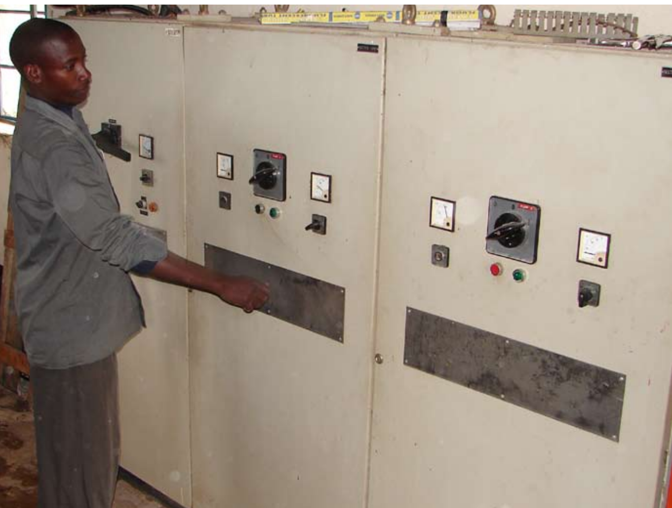
Booster house routing check. Photo © UN-Habitat
